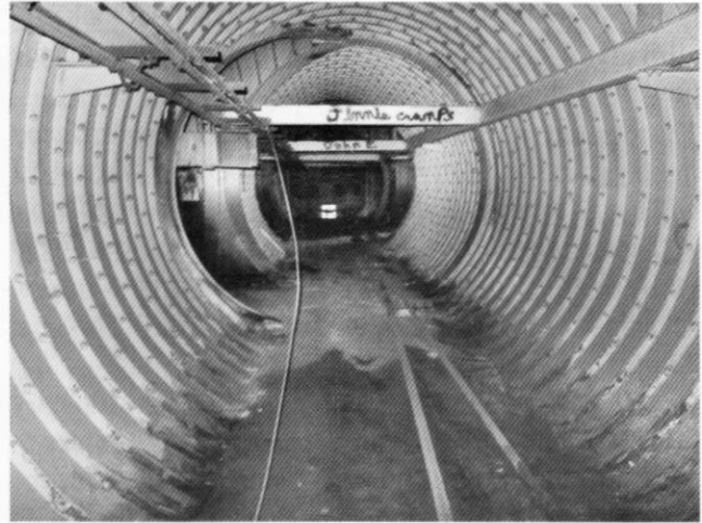
The exhaust tunnel. The diesel tanks are on the left and right in the middle. The exhaust shaft is visible in the distance
